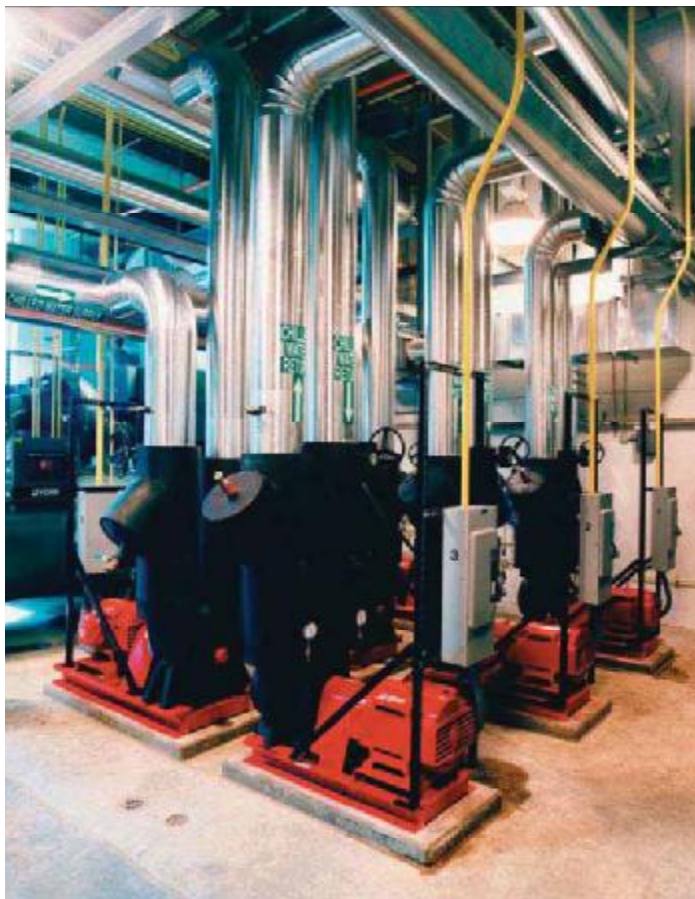
FIGURE 10.23 Photograph of Mechanical Piping
