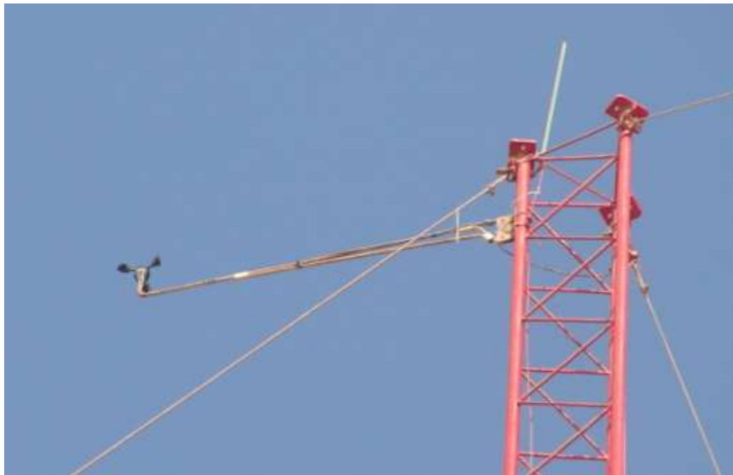
Figure 3.6: Top Mounted Boom Anemometer Installed on Green Power Mast
